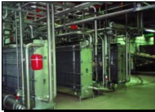
Pressure transmitter on line
