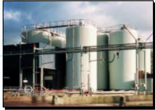
Level measurement on storage tanks
